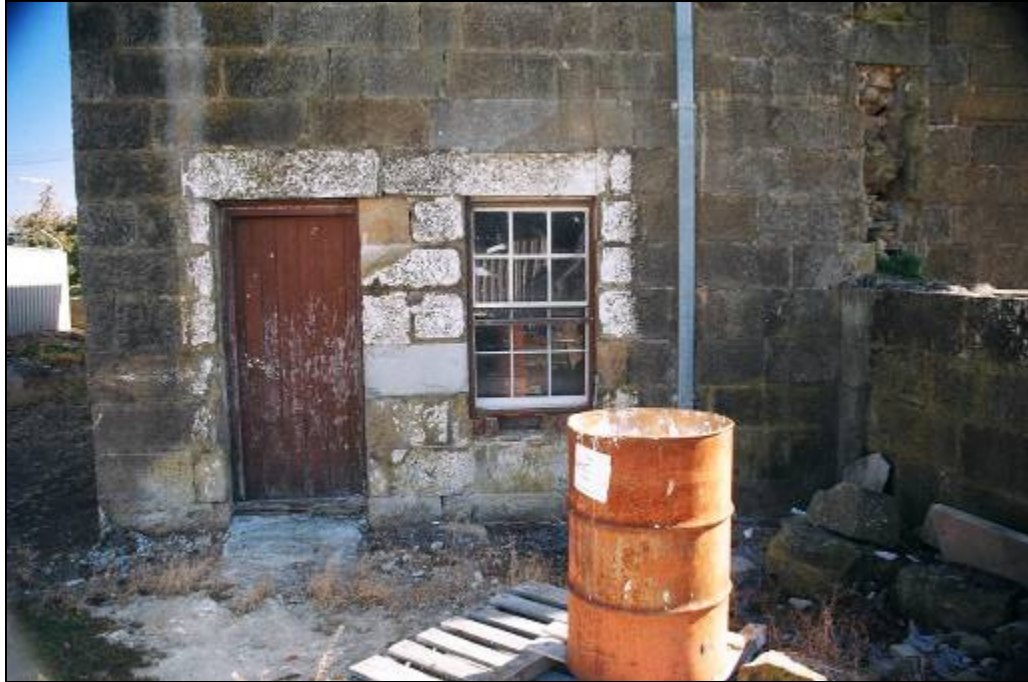
Plate 13.16 – Door leading from the eastern side of the Gaoler's residence (former men's kitchen) into the Outer Yard.
