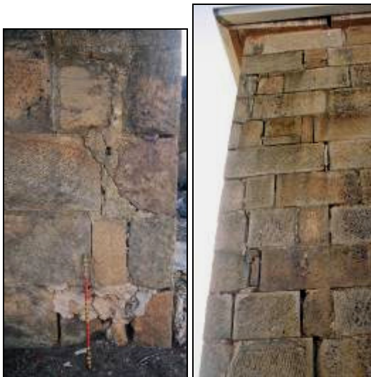
Plates 13.6 and 13.7 – Repaired scars on the south-eastern (left) and south-western corners of the Gaoler's residence from removal of the walls enclosing the Gaoler's yard.
