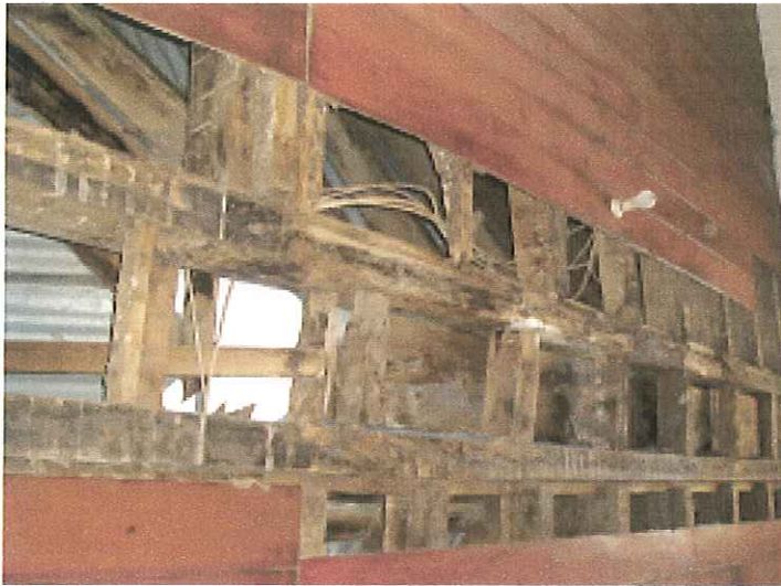
Photo 6. Rot of ceiling tie beams with water entry. A supporting wall has been removed increasing beam span and deflection.
