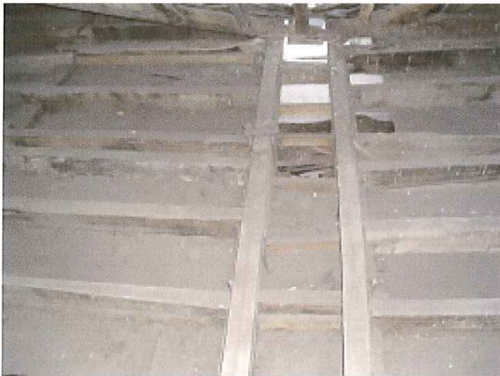
Photo 7. As photo 6 from above. The beam deflections have dropped the ends of the joists which the beams support.
