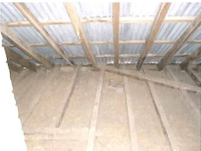
Photo 5. Note the very slender roof members which readily deflect or buckle in compression. Compression member span divided by member minimum thickness should not exceed 50.
