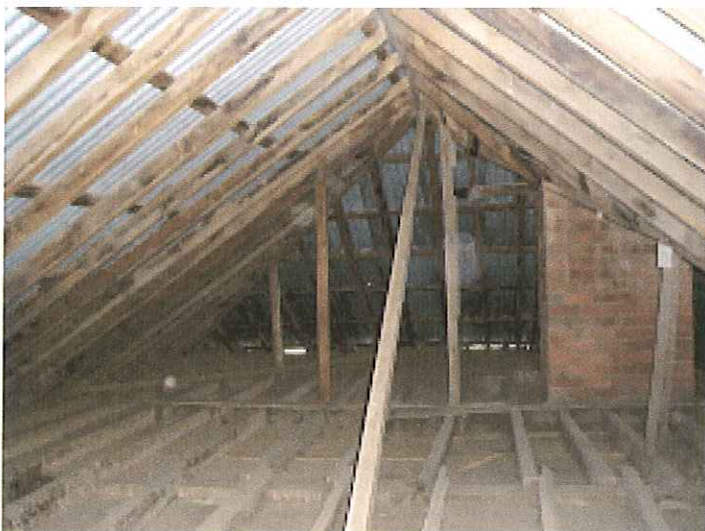
Photo 8. Typical roof construction with inadequate ridge support, readily buckled struts and braces and with all roof timbers undersized.
