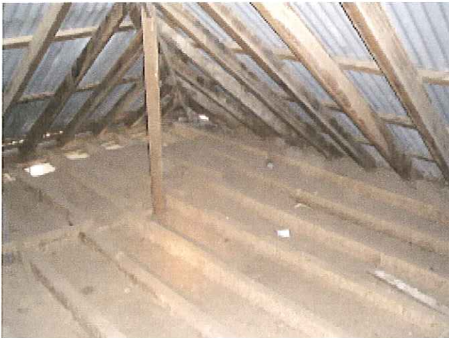
Photo 4. The roof lands on the outside ashlar. Note the joists on the right are parallel to the wall plate and there is no connection between the roof and the joists.
