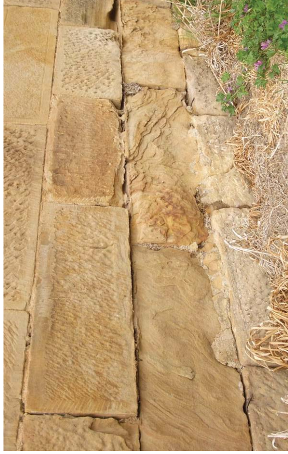
Severe deterioration of sandstone through ingress of chlorinated water.
