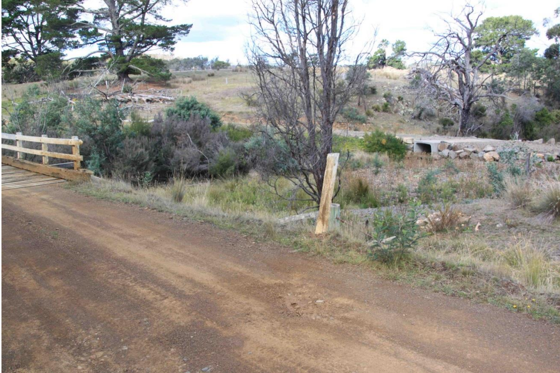
Heavy vehicle bypass culvert from the west abutment of the Swanston Bridge.
