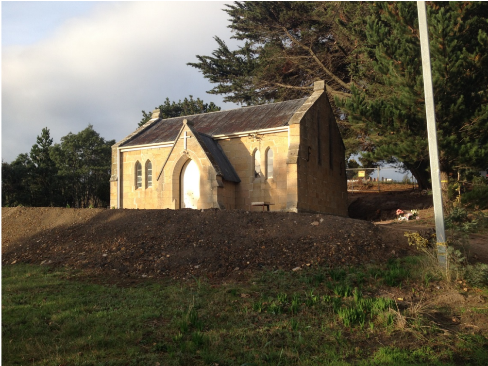
Photo 4_Photo demonstrates the fill and a possible car parking space on the 'Church Lane' side of St Anne's.
