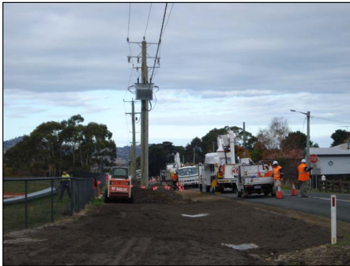
The new constructed swale in Reeve Street Campania, note the swale grated pits.
