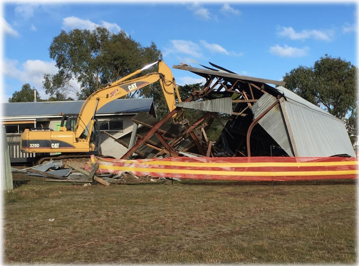
Demolition of the "condemned" Parattah Recreation Ground grandstand removes a dangerous structure from Council's building register
