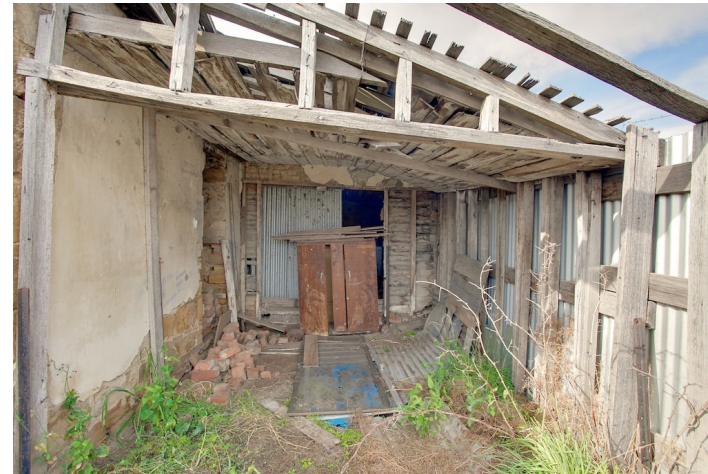
Pre-1845 timber skillion of the commissariat – one of the earliest timber buildings in Oatlands (Photo A. Bewley).
