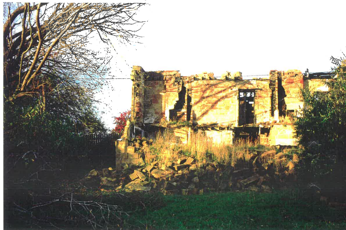
Unsafe stone wall.
