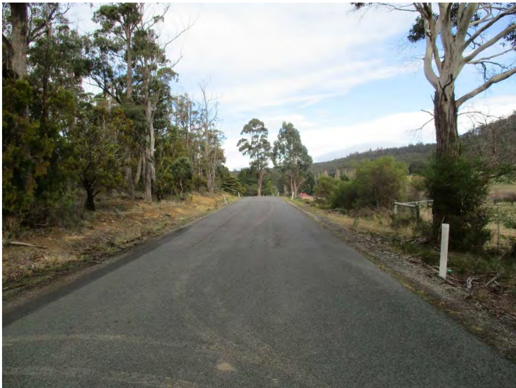
Photograph 6.4: View to south along Woodsdale Road from rear of vehicle turning right into the southern driveway
