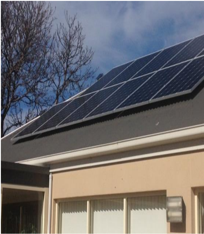
New Solar Panels at Councils Kempton Office
