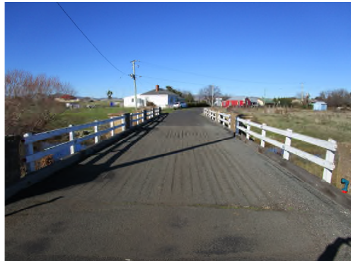
Photograph 7. View of deflected longitudinal deck planks with deflections due to wood rot .It is likely all of the bridge timbers require replacing. The longitudinal planking is a visual indication of how the bridge was constructed.
