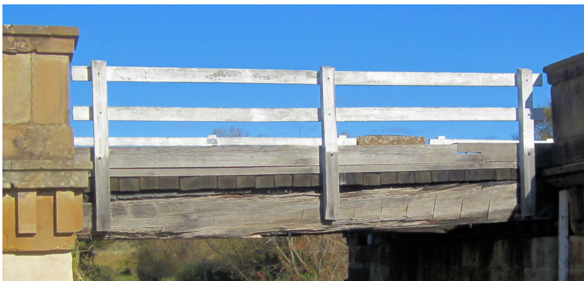
Photograph 8. Side view showing how the bridge was constructed. This is girder bridge construction.
