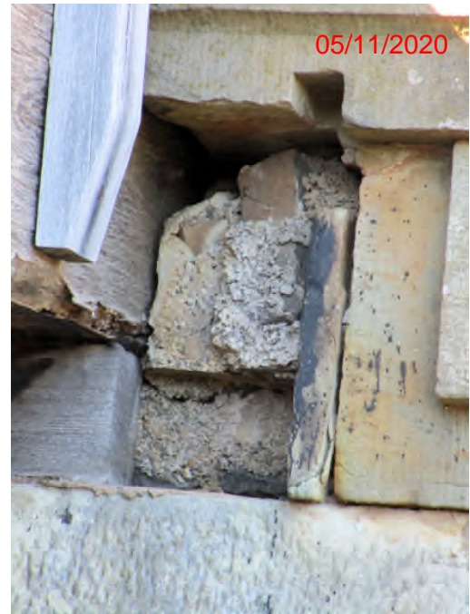
Photograph 6. View of log landing onto pier. The post support has partially been removed and the later work with concrete, likely inserted when the deck was raised, is not supporting the post.
