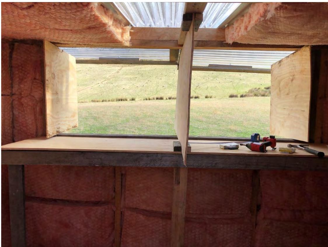
Figure 3 – Portable firing shed looking to the west of the site. A double layer of insulation batts is installed for noise elimination.
