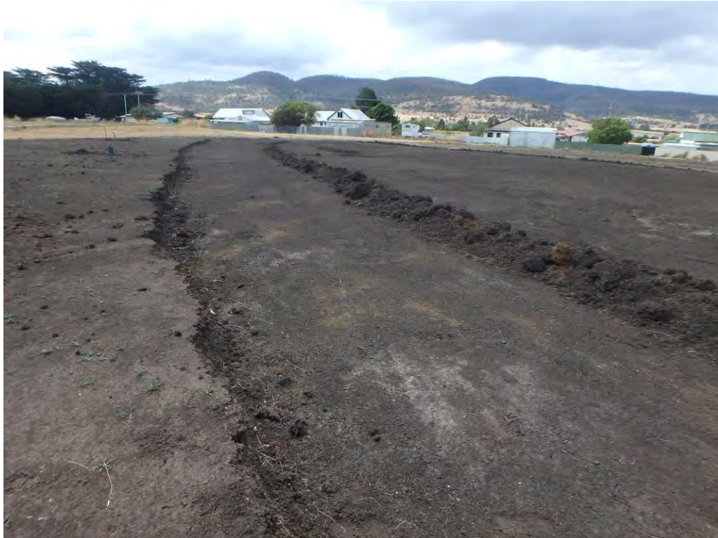
Plate 6: View north-east across the more heavily disturbed parts of the horse arenas footprint, with top soils stripped away to a depth of 30cm
