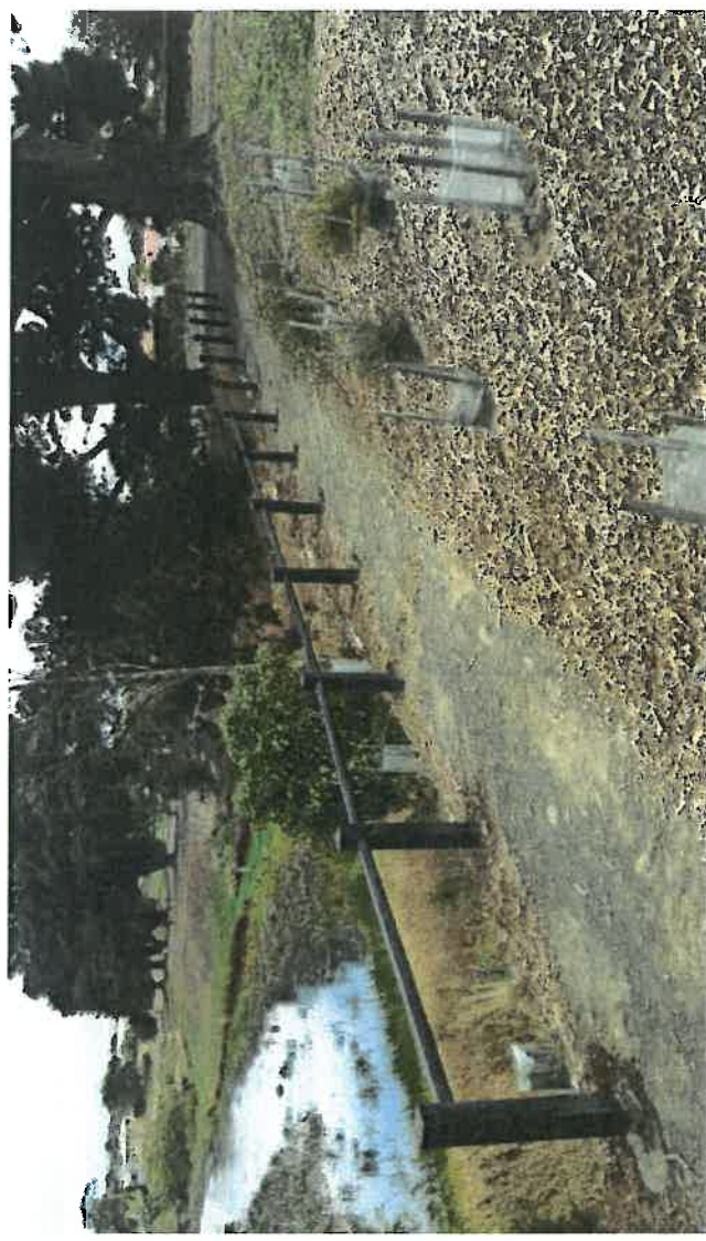
March 2017 – railing (recycled plastic) installed for added safety at the top of a steep bank section of the walking track (1 of 3 lots installed)
